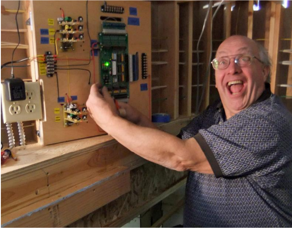
Actually, this is the new S-MINI board and related wiring in the "Medco Hole". If you guessed "B", you're correct.
