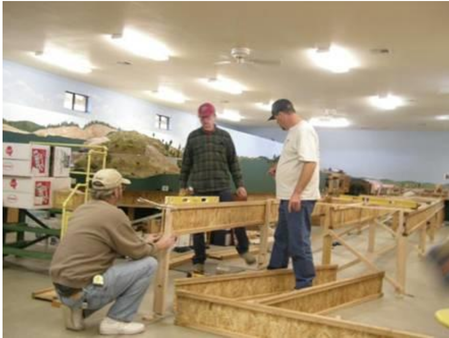
Part of the construction crew (Larry Tuttle, Brad Fawcett and Paul Konig)
