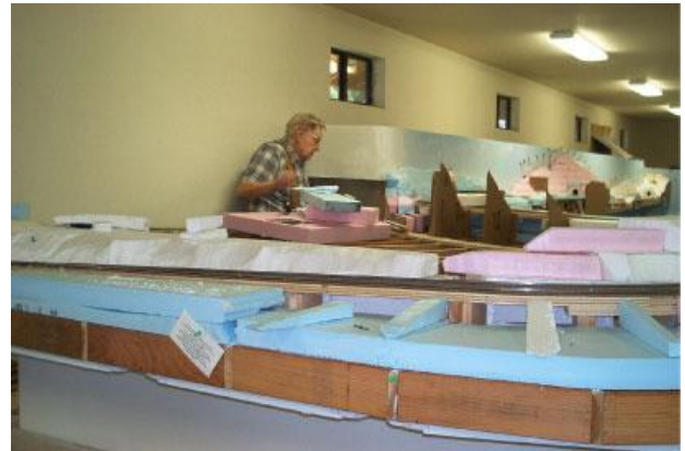
Wil Cleveland works inside the Cascade Crest installing a curved scenery backdrop
